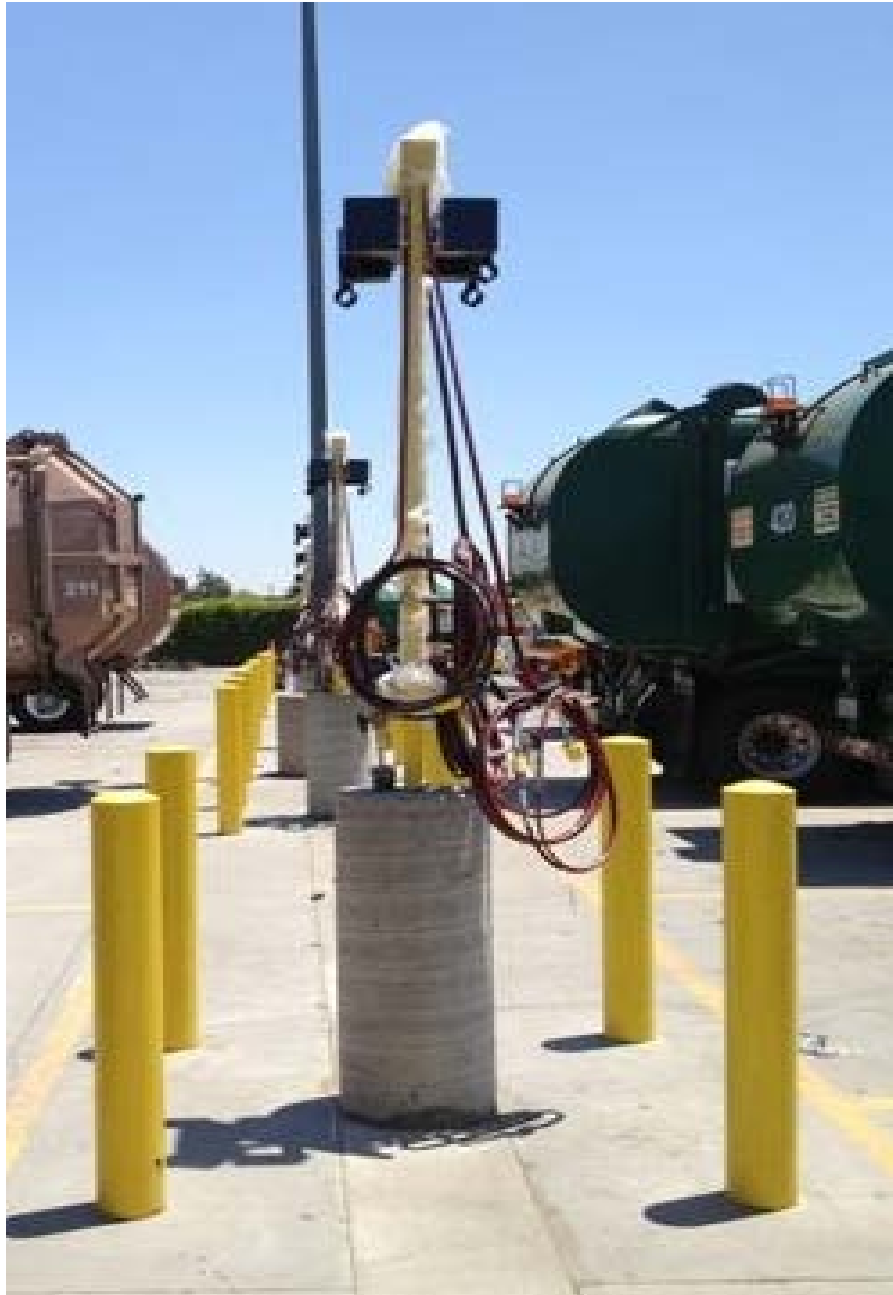
Slow Fill Dispenser
