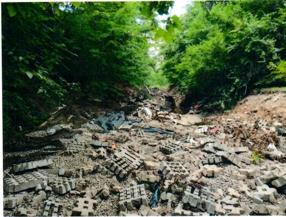
Damaged Area of the Channel
