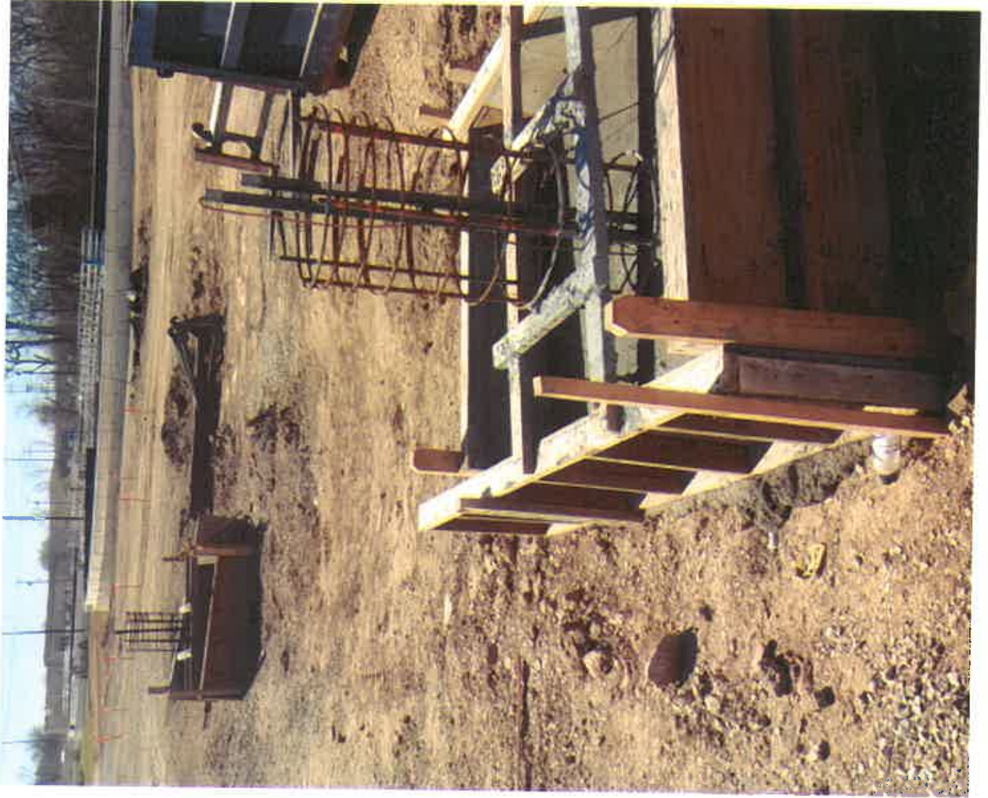
Excavation reduced from 4 hours to 2 hours per base. Photo is an example of bases that did not require any excavation.
