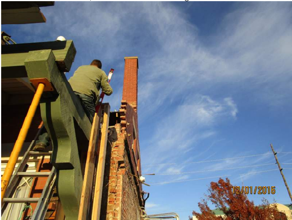
Photo 8 – December 1, 2016: Chimney at South Wall Leaning to South
