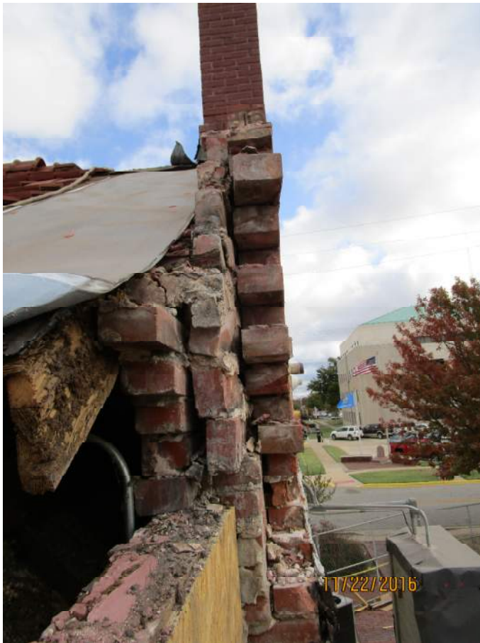
Photo 6 – November 22, 2016: Damaged Rafter at South Gable Exposed
