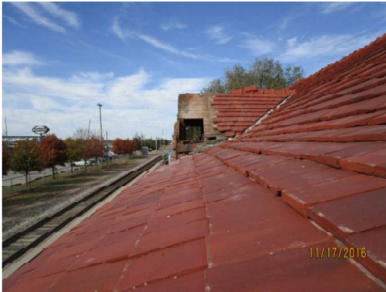
Photo 5 – November 17, 2016: Water Damage at West Gable
