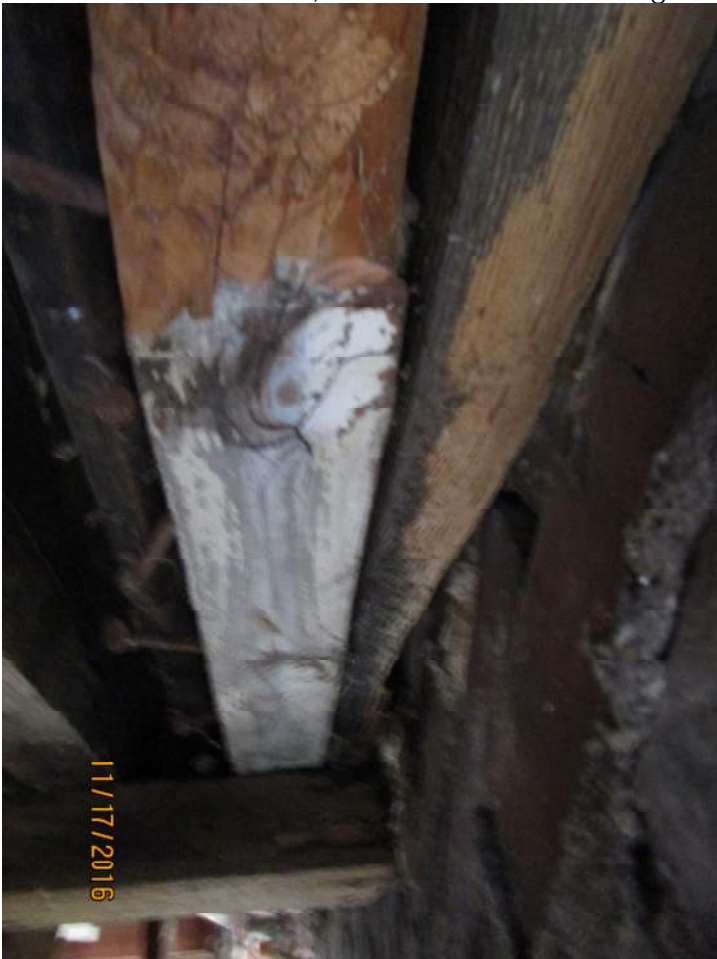
Photo 4 – November 17, 2016: Water Damaged Rafters at South Gable of Waiting Area
