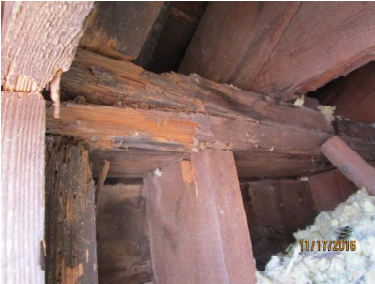
Photo 3 – November 17, 2016: More Water Damaged Studs Uncovered at SW Corner
