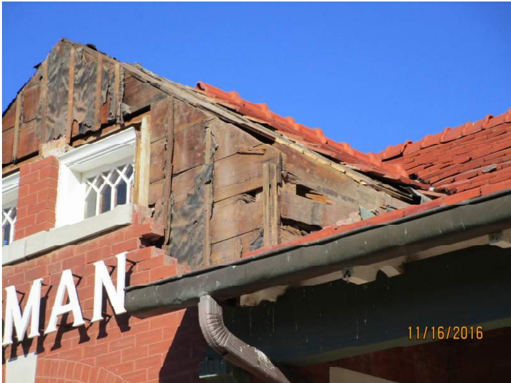
Photo 1 – November 16, 2016: West Gable Wood Damage Uncovered
