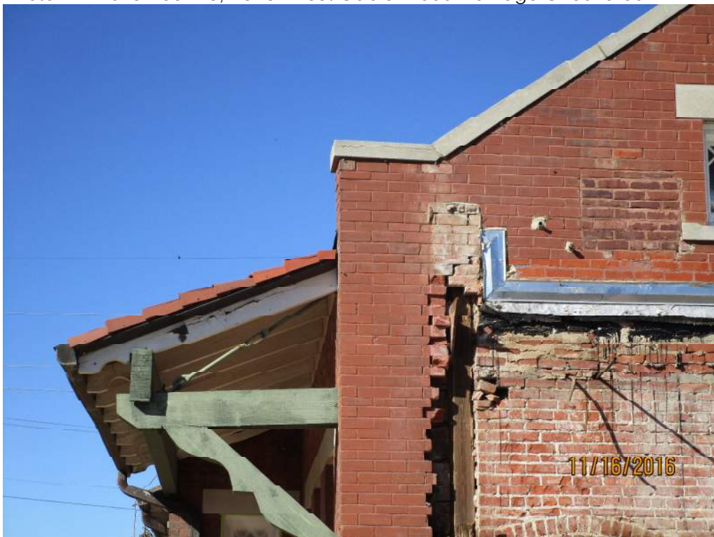
Photo 2 – November 16, 2016: Southwest Corner Water Damaged Stud Uncovered
