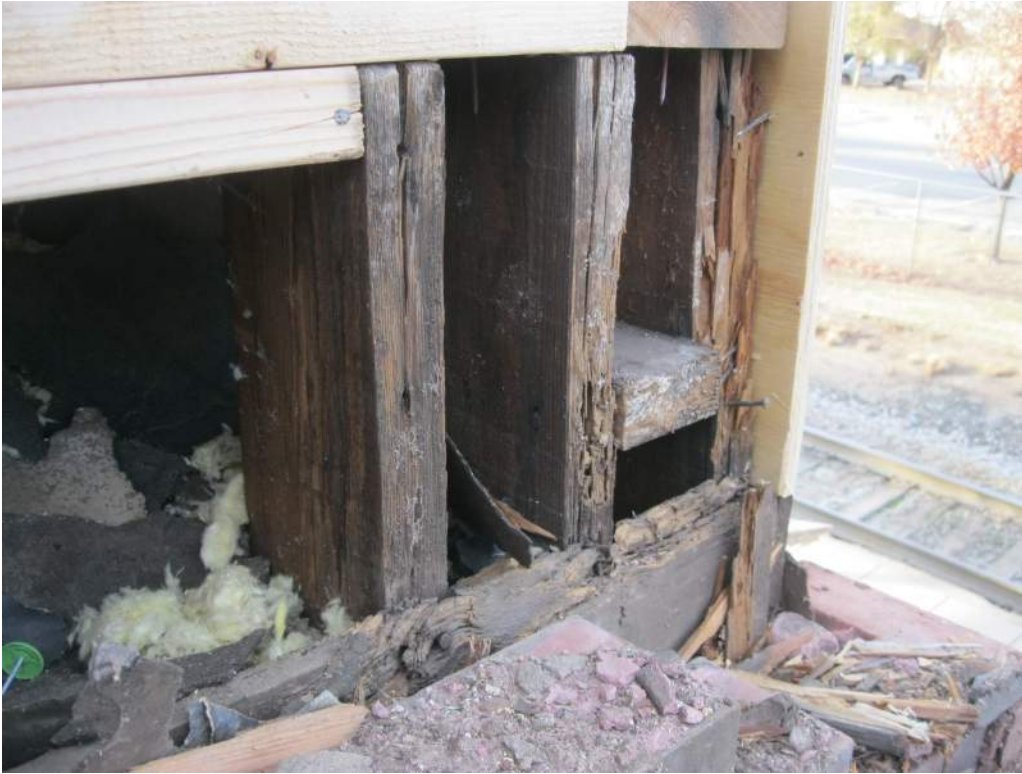
Photo 9 – December 2, 2016: Water Damaged Studs at NW Corner below West Gable
