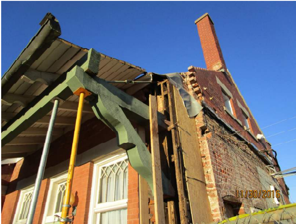
Photo 7 – November 30, 2016: SW Roof Overhang Bracket Not connected to Wall
