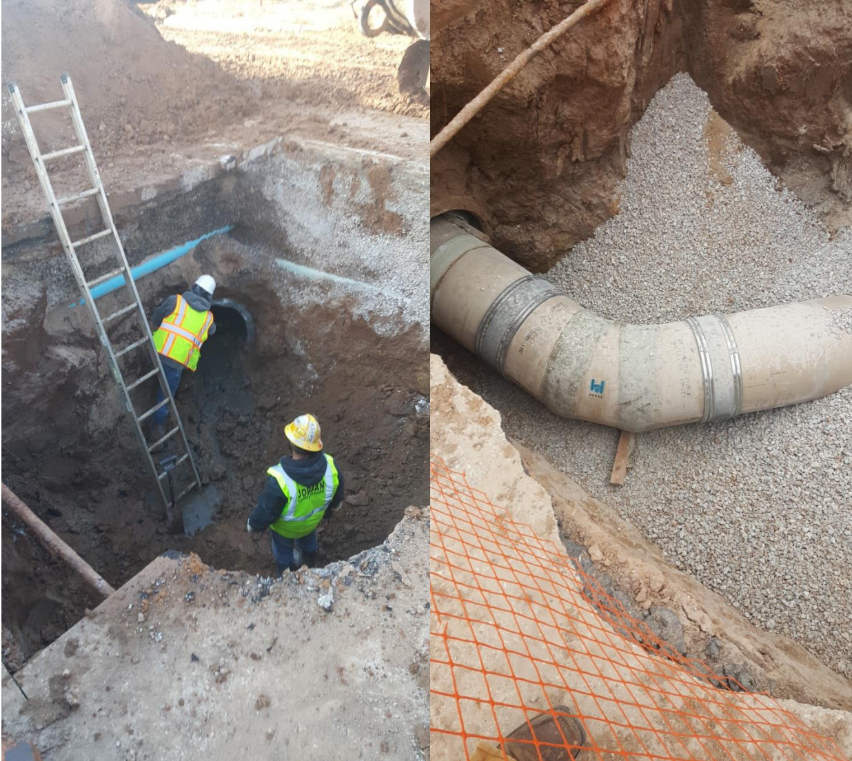
Before and after photos of new 27-inch FRP piping, fittings and Fernco couplings in roadway NE of Environmental Services Building on Influent Line to Primary Clarifiers 3 and 4.
