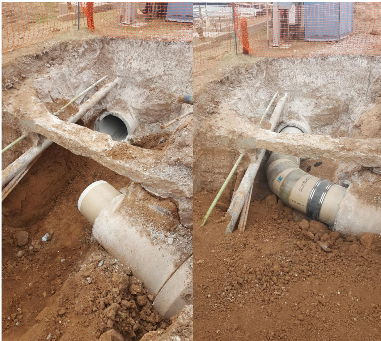
Before and after photos of new 27-inch FRP piping inserted in 30-inch RCP and fittings and Fernco couplings south of Motor Control Center on Influent Line to Primary Clarifiers 3 and 4
