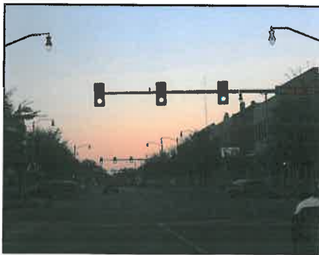
Coordinated signal systems provide bandwidth to minimize stops on arterial routes
