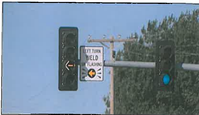
FYA signal heads have been installed on a city-wide basis
