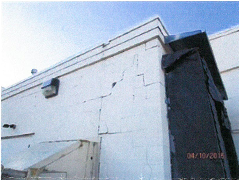
Document Name: Damage - 2.JPG
