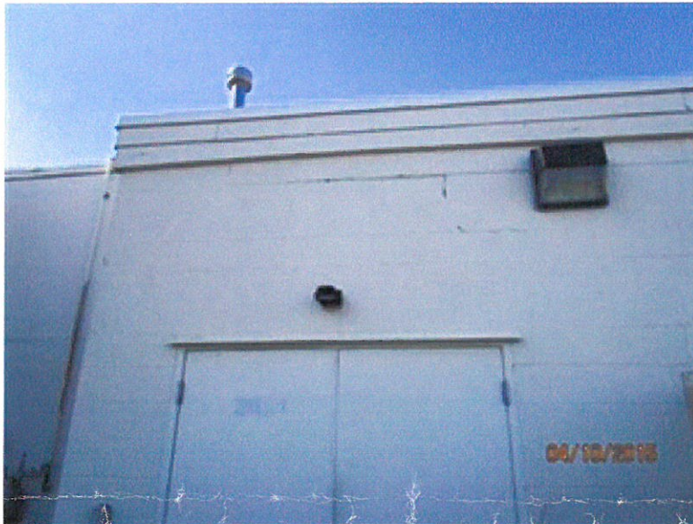
Document Name: Damage over the door.JPG
