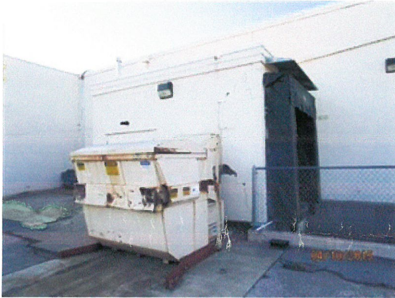
Document Name: view of damage.JPG
