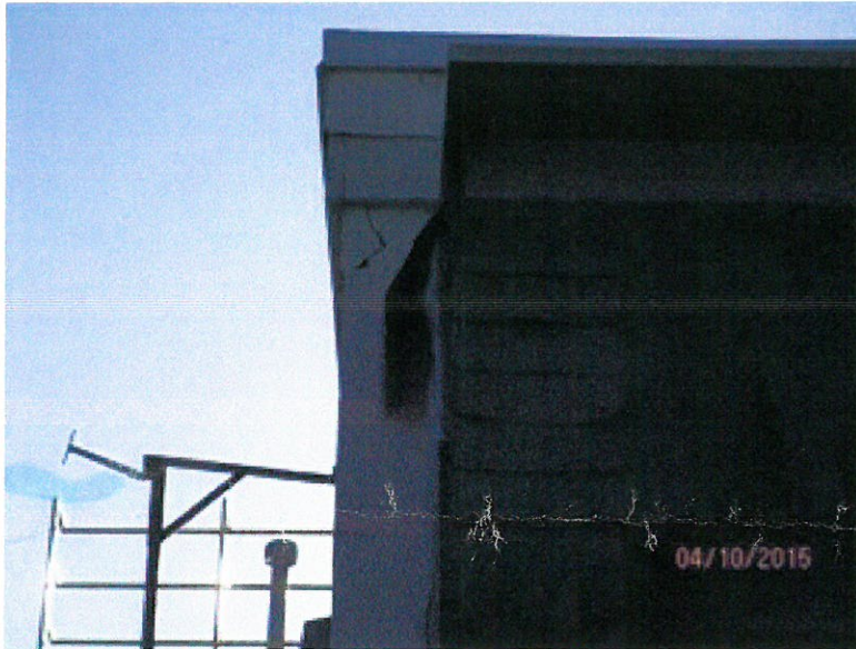
Document Name: Damage at corner.JPG
