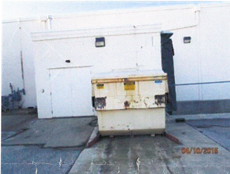
Document Name: view of damage - 2.JPG
