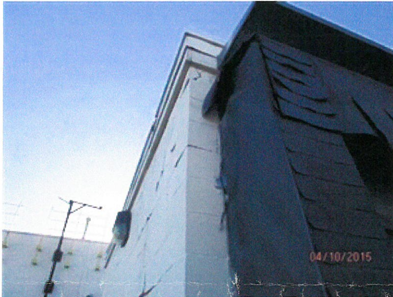
Document Name: Damage - 4.JPG
