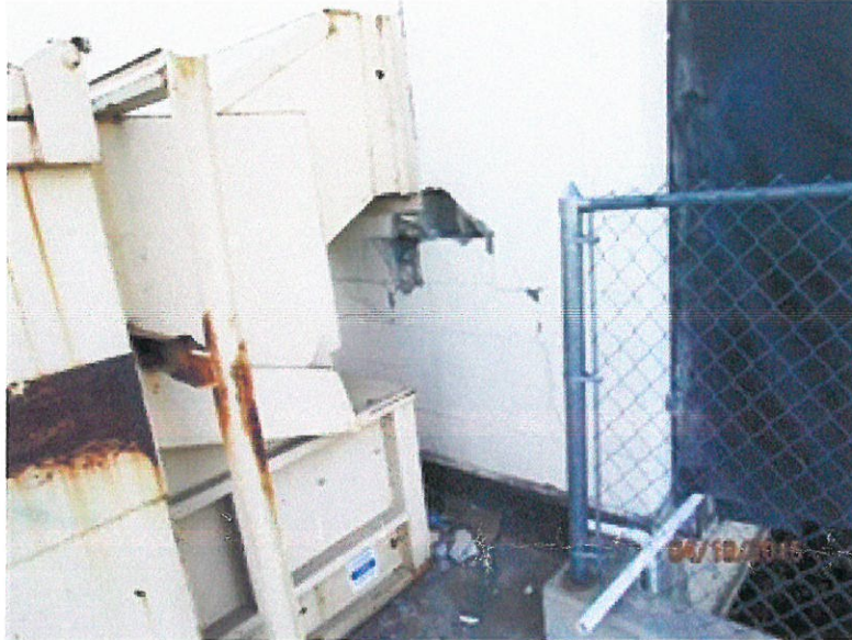
Document Name: Damage.JPG
