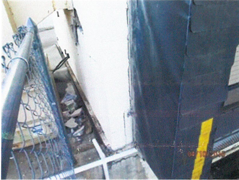
Document Name: Damage - 3.JPG
