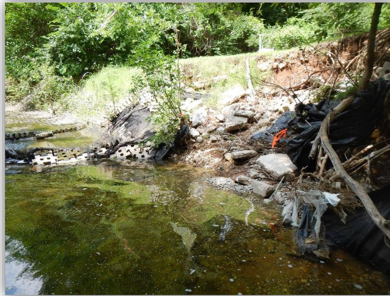
Figure 2: Articulated Block Channel Failure
